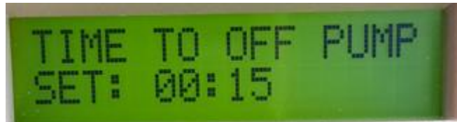
Fig.7. Time to off pump set panel
