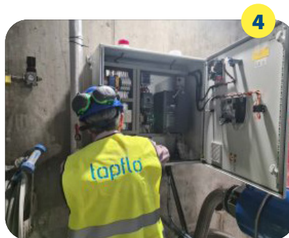
Control panel installation
