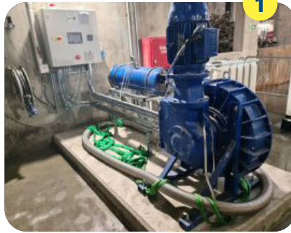
Phase two - installation complete with further supports, control panel, and unistrut cable trays
